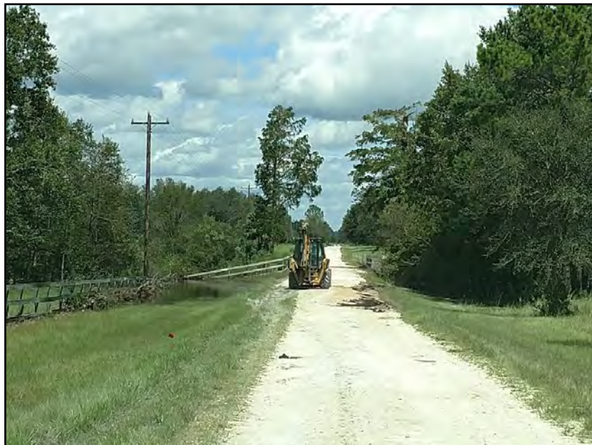
FWC Wildlife Biologist and Area Manager Jason Slater had to immediately go to work with this backhoe to fill in the large impassible holes in the road to allow other FWC employees and their families to be able to get out of their state housing on the property. Prior to being able to fill in the holes, FWC employees and their families had to scoop out hundreds of two-toed amphiumas ( Amphiuma means ) that were trapped in the holes! (Photo credit: Jodi Slater)
